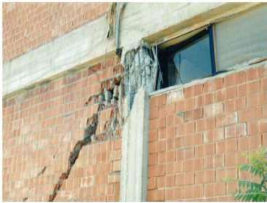
Figure 1.5: Short column failure [2]
